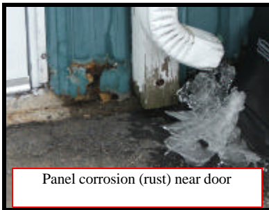
Panel corrosion south wall of building
